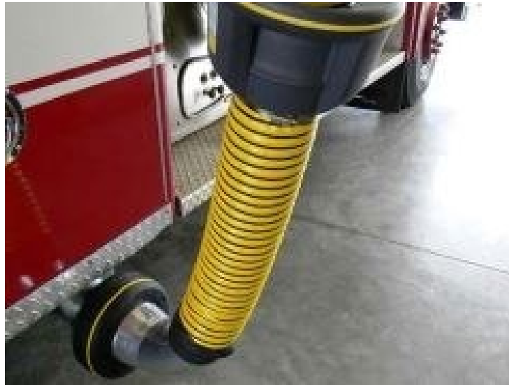
Figure 28. Source Capture Diesel Exhaust Extraction System
