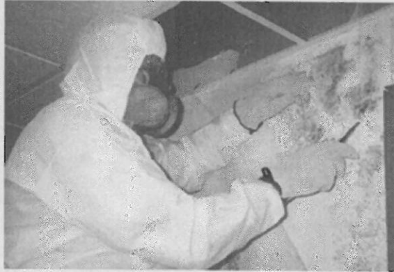
Photo 7. Remediation worker with limited PPE
