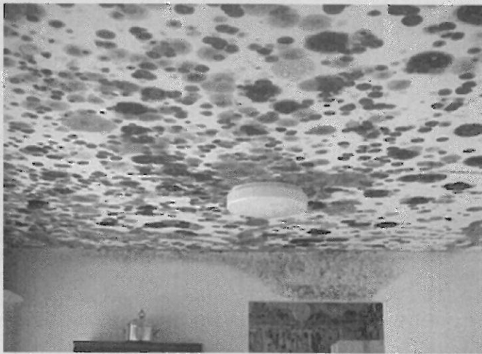
Photo 2: Extensive mold contamination of ceiling and walls
